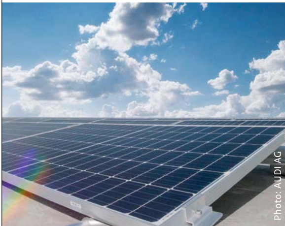
Audi Hungaria: photovoltaic system on the roofs of the two logistics halls.
