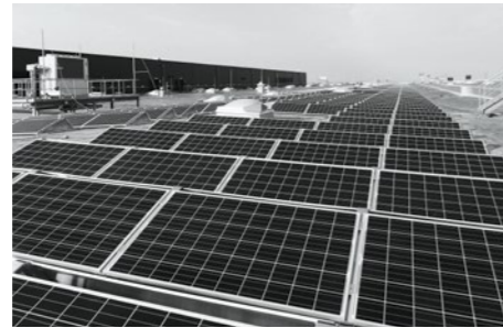
PHOTOVOLTAIC SYSTEMS AT LEIPZIG PLANT
